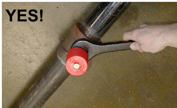
Figure 1: Correct use of designated installation wrench with ESFR Pendent K14 Sprinkler SIN VK500 and sprinkler cap
