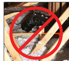
INCORRECT (Exposed piping)
