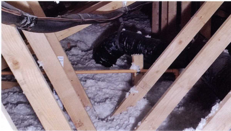
Exposed Piping: Sprinkler system piping should not be left exposed in unconditioned attic spaces.
