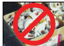
INCORRECT (Protective caps not in place)
