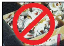
INCORRECT (Protective caps not in place)
