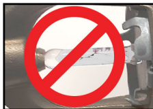
INCORRECT (bulb cracked, fluid missing)
