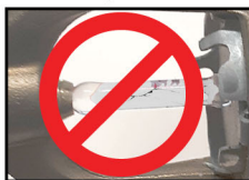
INCORRECT (bulb cracked, fluid missing)
