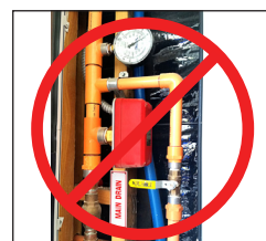
INCORRECT (No pressure relief valve)
